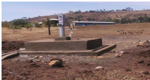
The newly constructed potable water point in school of Anena
